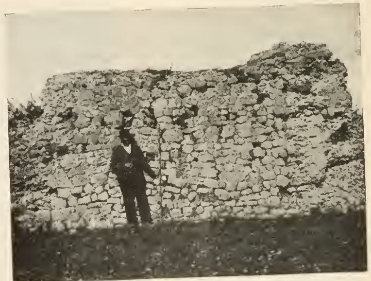
4. A PIECE OF THE MURO PERTUSO BETWEEN TWO BUTTRESSES View from the south
